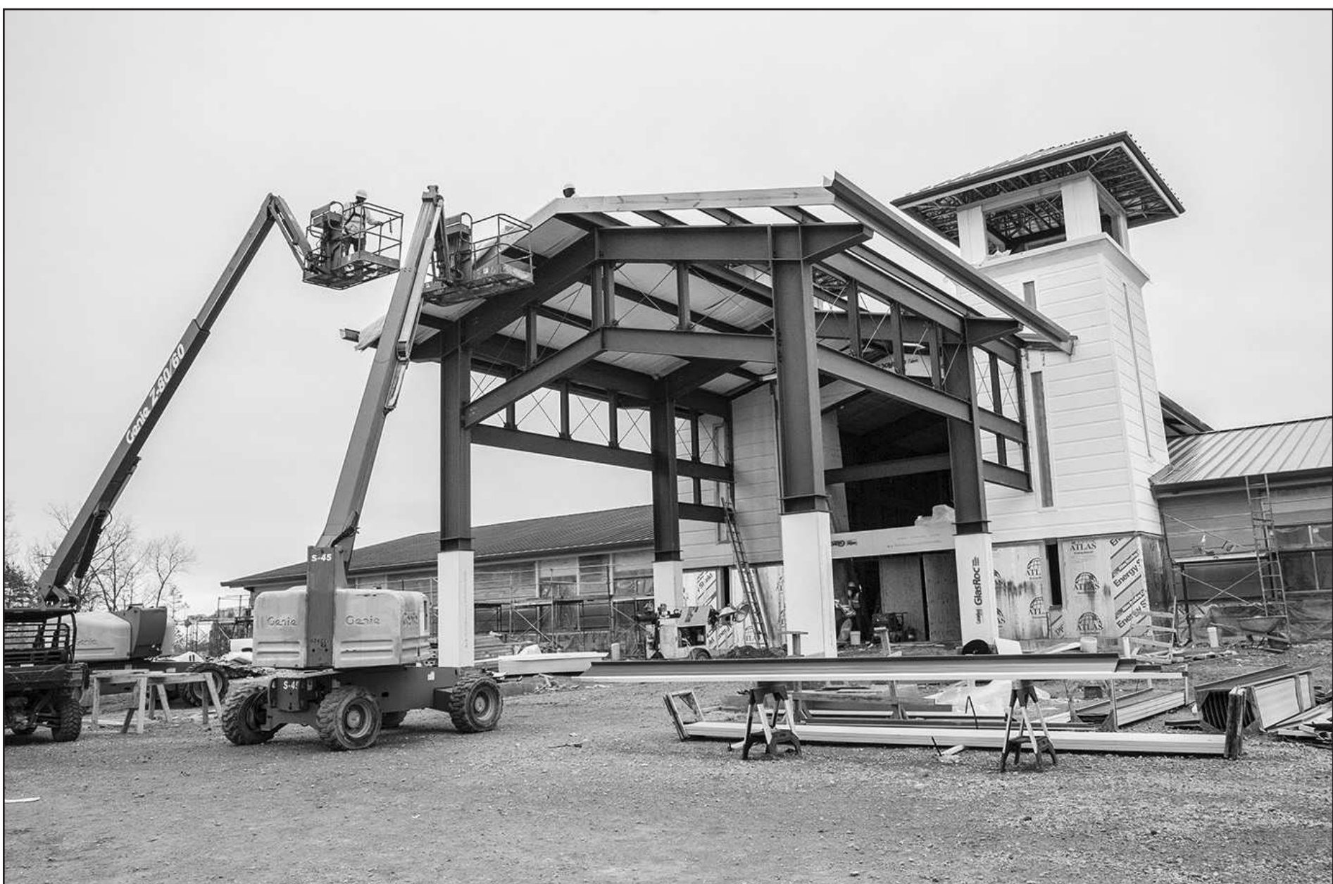
Rabren General Contractors Inc. from Auburn has handled the construction of the marksmanship park. The earthmoving phase began in December 2013, and construction continued throughout last year. The facility is set to open in May.
